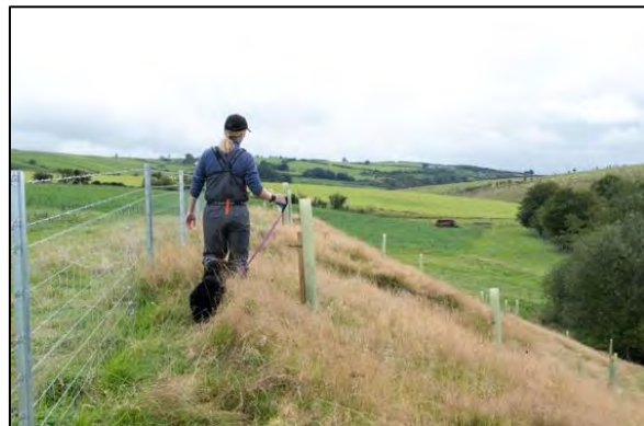
The Clipex Fencing has been installed on this (the right) bank and broadleaf trees have been planted throughout the protected area.
