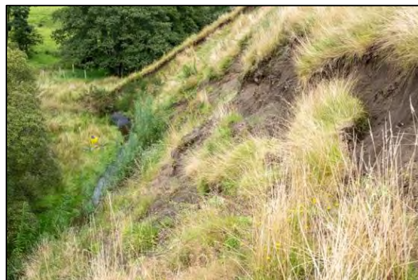
After: Much of the slope is now vegetated and the green engineering on the riverbank is visible and growing rapidly.
