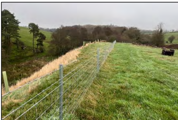
These metal clipex fencing systems should out last traditional timber fences and are somewhat quicker to install in ground free of stones.
