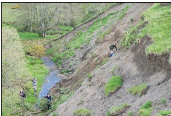
Before: ART staff and volunteers planting willow and sewing wildflower and grass seed across the eroding bare slope before installing green engineering.
