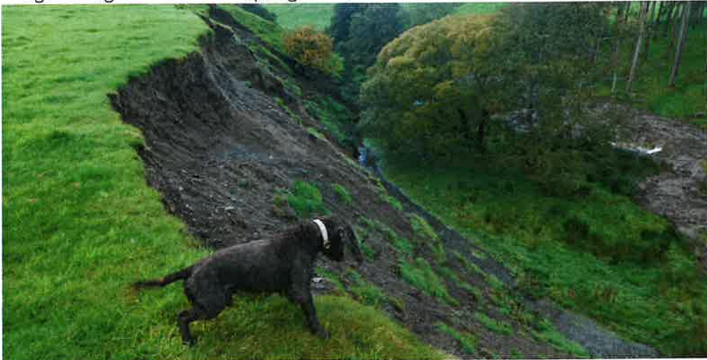
Severe landslide causing heavy siltation in the Netherton Burn. This entire area will be fenced to exclude livestock
