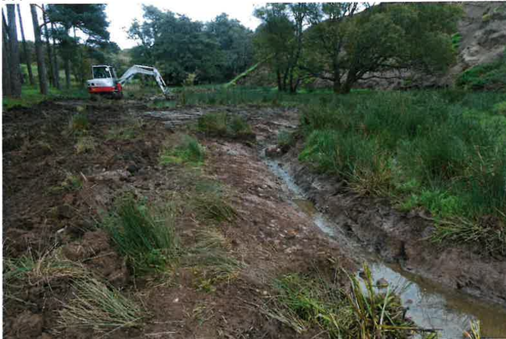
Creating a new 'wildlife channel' that will carry water during high flow events thus reducing pressure on the landslide.
