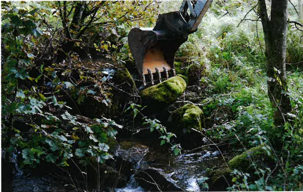
Removing the old weir that prevented fish access to the upper reaches of Netherton Burn
