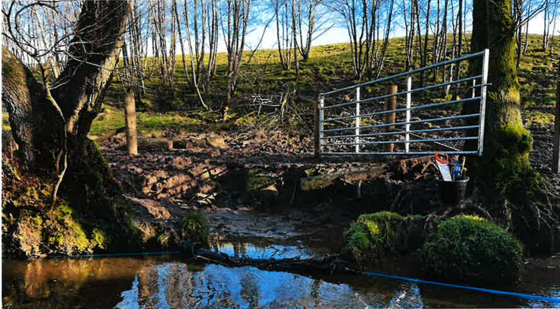
Newly installed fencing and gate in severely degraded salmon habitat on Brockloch Burn
